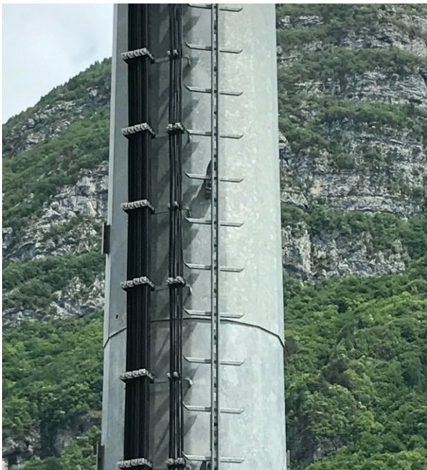
Fall Safe Ladder on Pole
