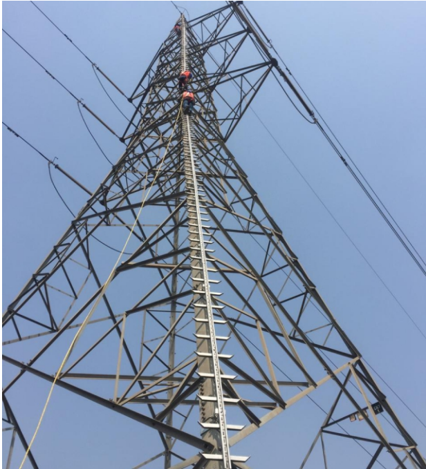
Fall Safe Ladder on Transmission Tower
